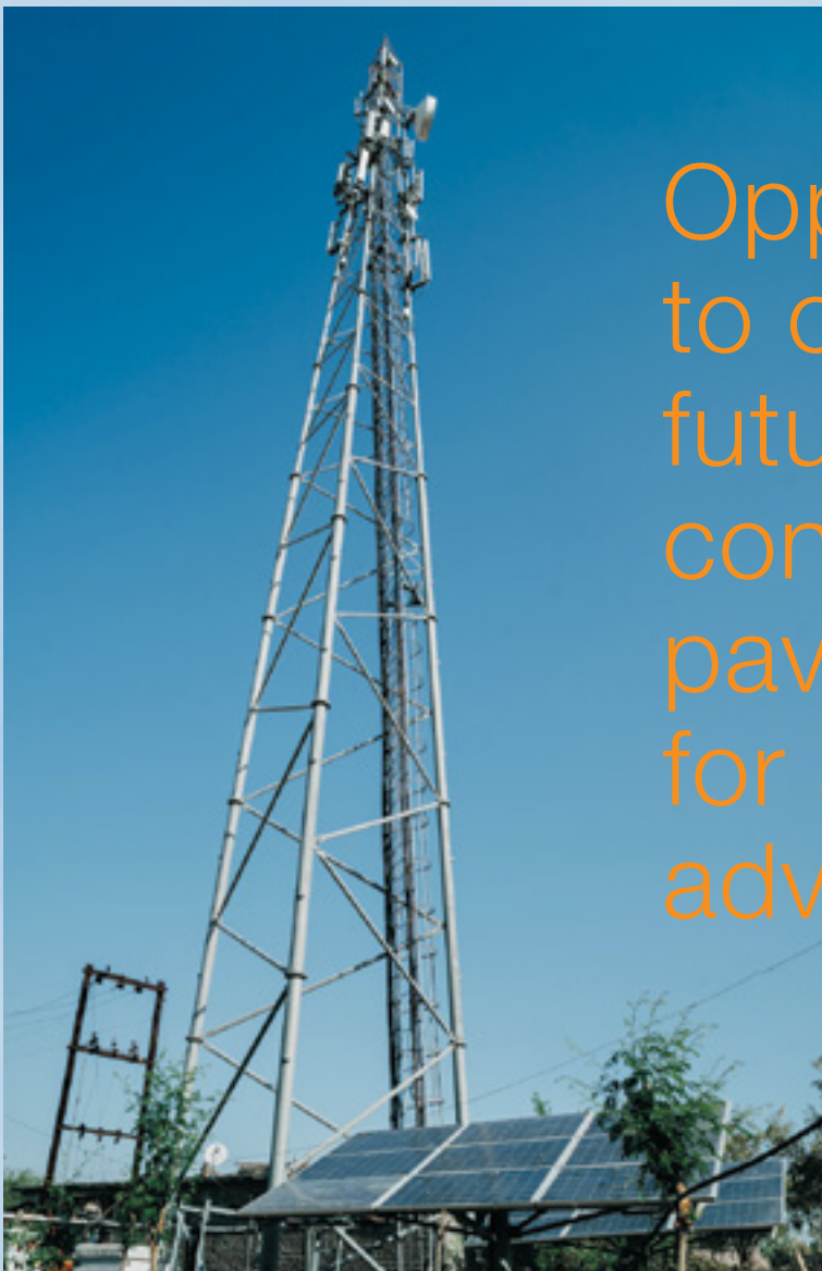
↑ Solar energy enabled telecom tower at Sehore (near Bhopal)
