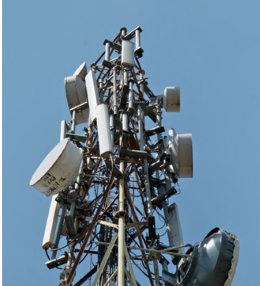
↑ Telecom Tower at Bhopal
